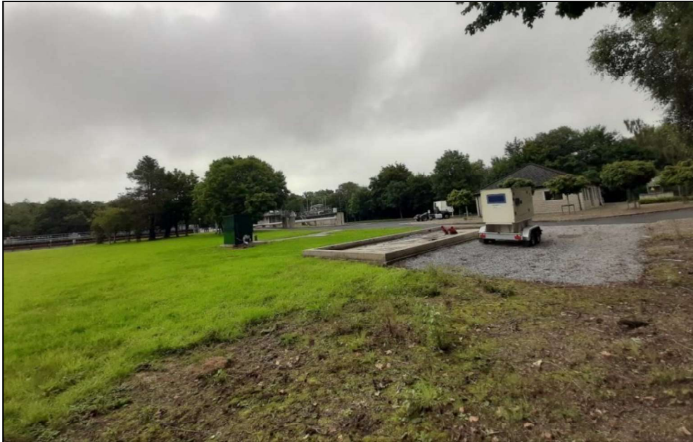
Figure 11-3: WwTP infrastructure classified as buildings and artificial surfaces (BL3) and associated hard stand areas of (BL3)/spoil and bare ground (ED2)/recolonising bare ground (ED3). Grassland classified as amenity grassland (GA2).
